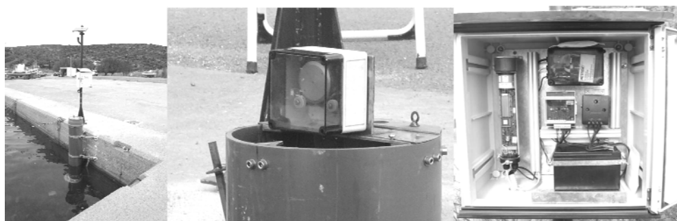
Figure 4. Left: The instrument with the solar collector in operation – Middle: The recording instrument fixed on the pipe – Right: The recording unit, the modem, the transformers and the battery.
